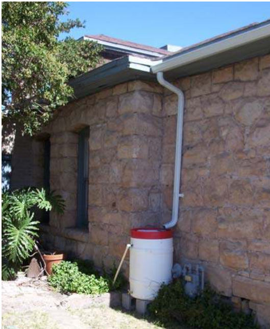
Water harvesting system in Nogales, Arizona
